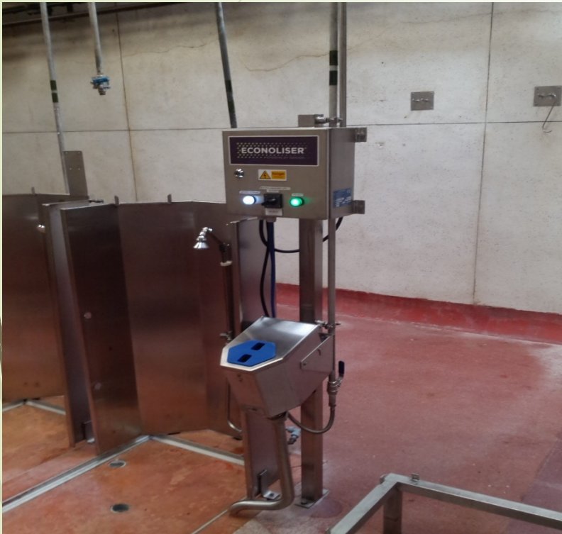
Application of Econoliser in a beef packing a plant
